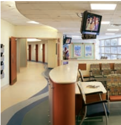
left: Tampa General Hospital from top: Mass decontamination showers have the capability to decontaminate up to 200 patients per hour with quick-connect plumbing pipes from above. Medical gas cabinets throughout the corridors, waiting rooms and offices increase capacity in the event of patient census spikes.
